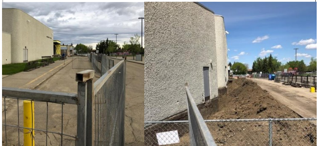
Right: Though there remains much work to be done on the school addition, the fencing around the existing building is a sign that work is transitioning from construction to renovation. This here is a before the backhoe picture and after
