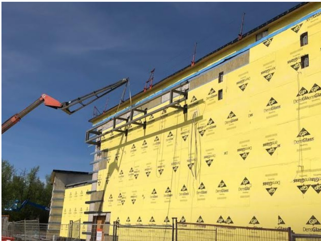
Bottom Left: Welders install the metal 'eyebrow' on the east side of the 'old' gymnasium. The eyebrow is an aesthetic feature which will compliment the brick and metal cladding/siding.
