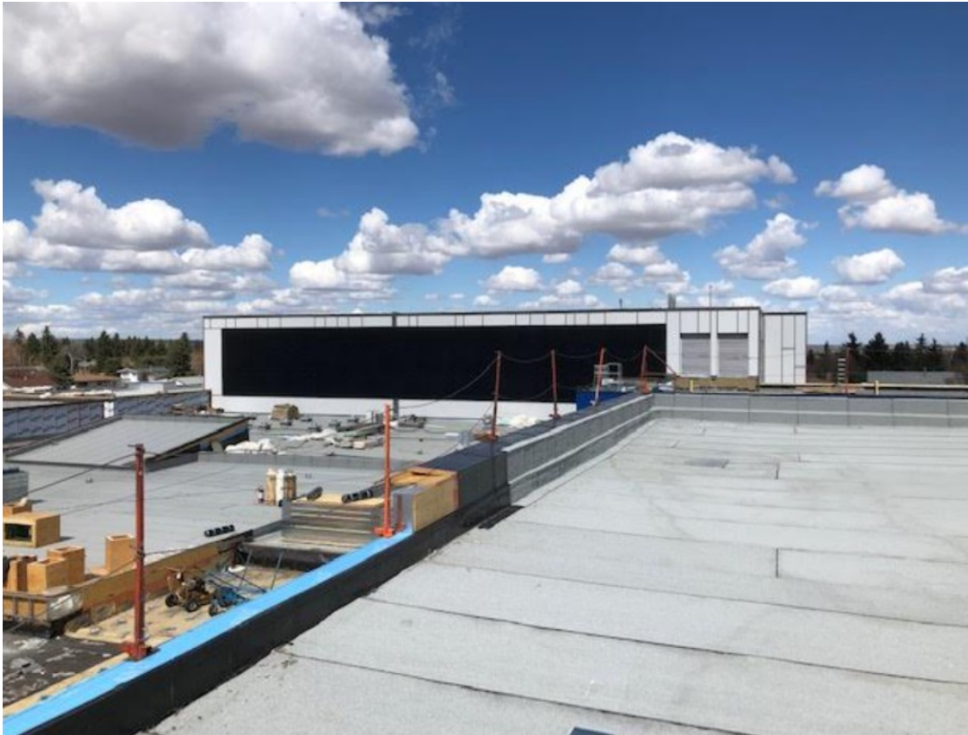
Top Left: A photo of the solar panels on the south side of the new gymnasium taken from the newly renovated roof of the old gymnasium.
