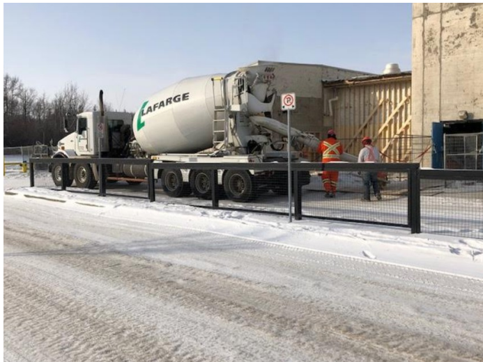
Bottom Left & Right: A cement and pumper truck arrive after the February cold snap to pour the flooring in the old office space and the old Phys. Ed offices and change rooms.
